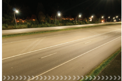
Black Lake Adaptive LED Lighting System on State Highways project | Photo courtesy WSDOT
