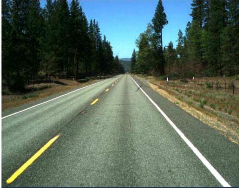
Figure 6-2. A photo of the asphalt concrete overlaid JPCP taken at PM 24.6 NB of the Weed project.
