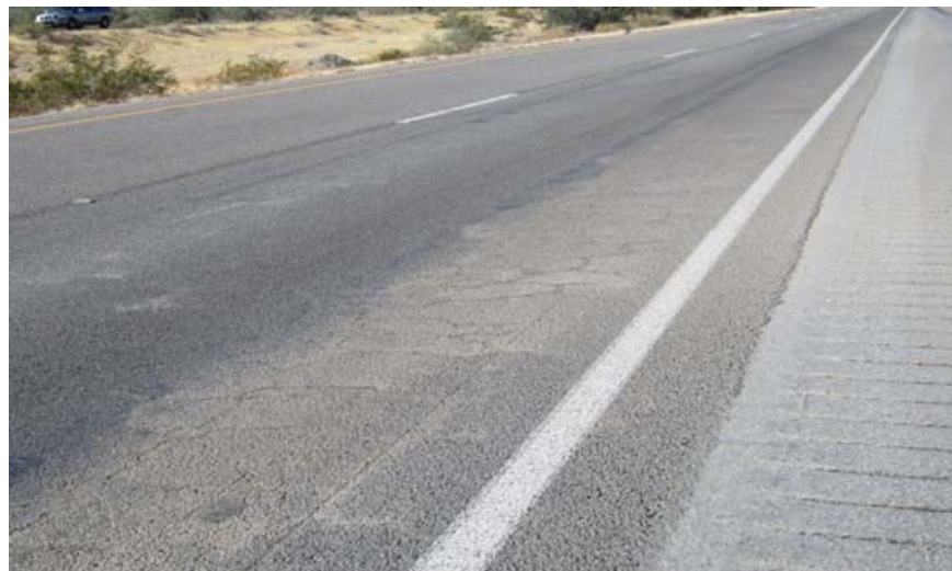
Figure 9-3. Photo showing pumping in the fatigue cracked wheel path taken at PM 104 Eastbound.
