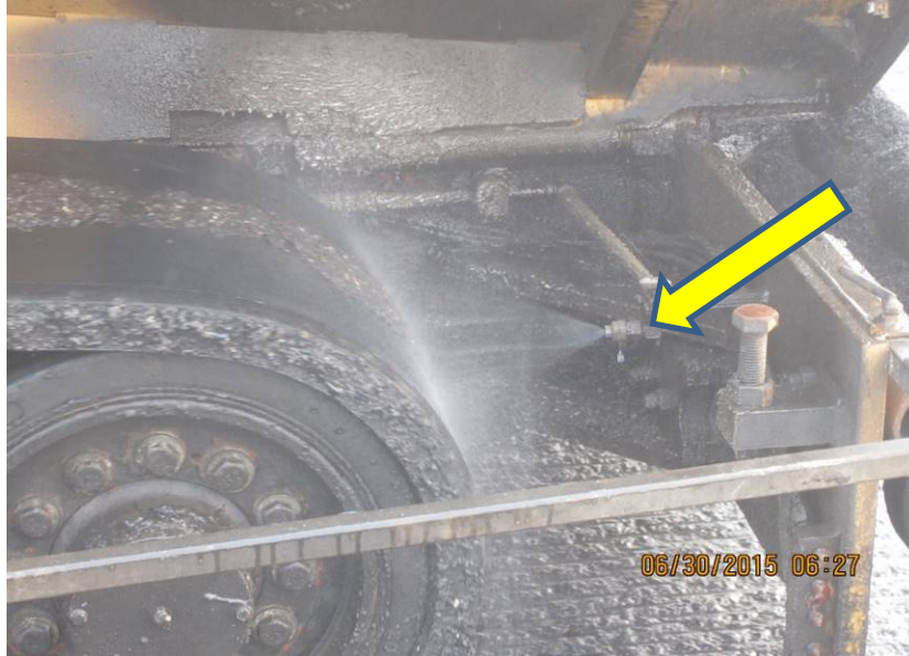
Figure 13. Water Nozzle Installed in Front of the Rubber-Track to Reduce Mix and Tack Coat Pick-Up along the IL 116 Project
