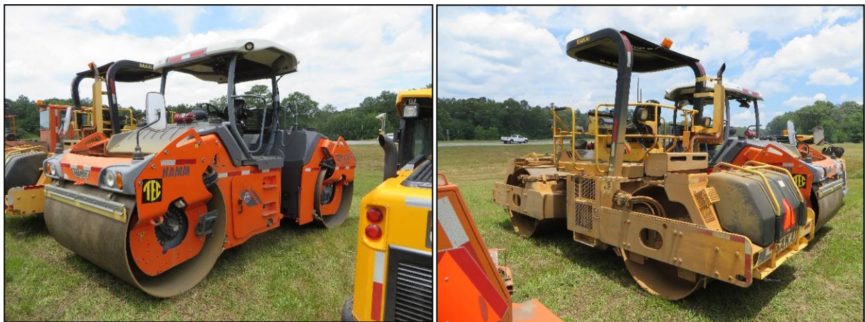
Figure 5. Hamm Roller Used in the Breakdown, and Sakai Roller Used in the Finish Rolling Position to Compact the Asphalt Concrete Mixture.
