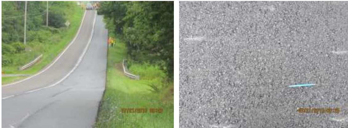
Figure 8. Roller Marks (photo on the left) and Checking (photo on the right) that Occurred in the Northbound Lane within the Temperature Sensitive Zone of the Mixture (see figure 7)
