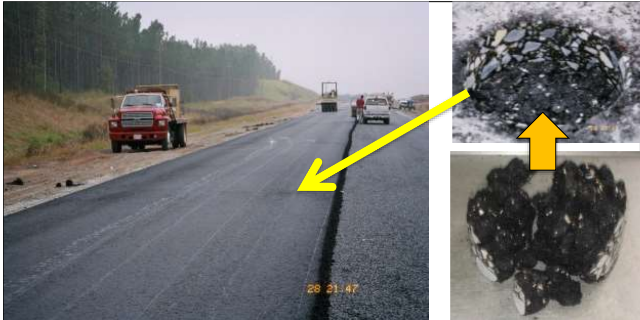
Figure 2. Truck to Truck and Longitudinal Segregation
