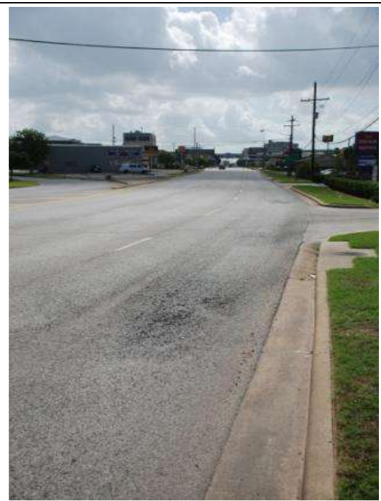
Figure 12. Raveling of the Wearing Surface from a Cold Spot during Construction.
