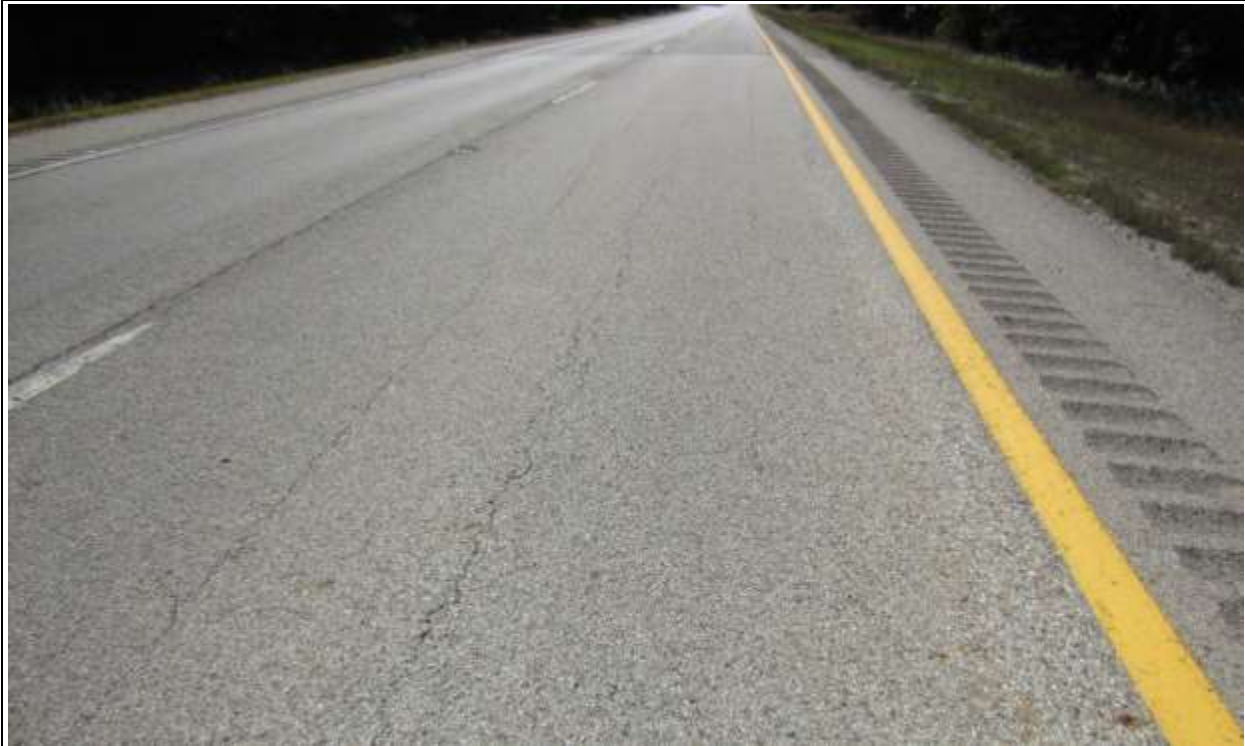
Figure 11. Longitudinal Cracks from Thermal Streaks during Construction.
