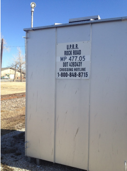
Figure 3-1: DOT Number Postings at Grade Crossings ENS Sign (Left) and Railroad Signal House (Right)
