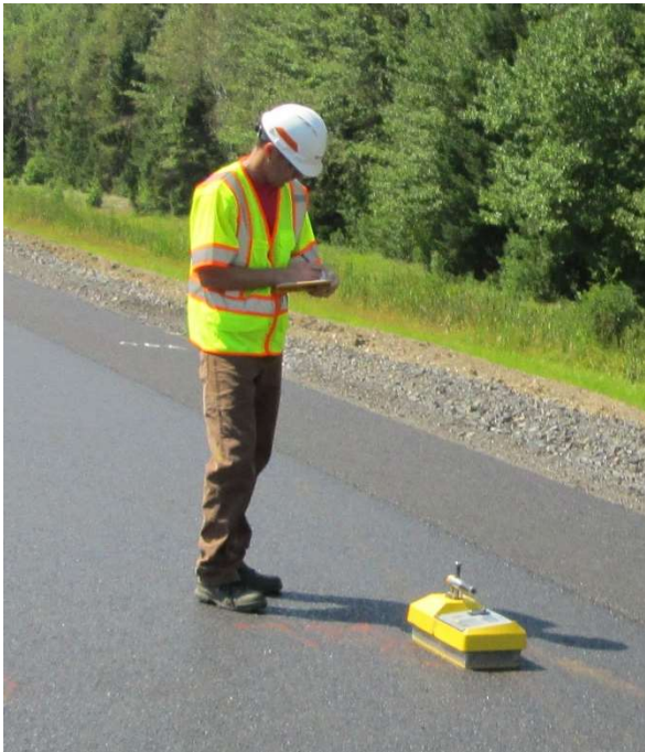
Density gauge (Nuclear or electrical)
