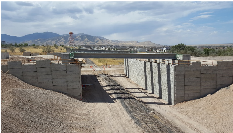
For the Mountain View Corridor project, the finished girder placement is over the Bacchus Spur, owned by UPRR.
