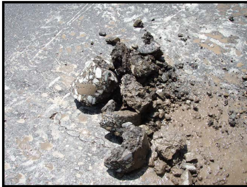
Figure 3.9: Signs of “Stripped” AC Layer on I-10 (WB)
