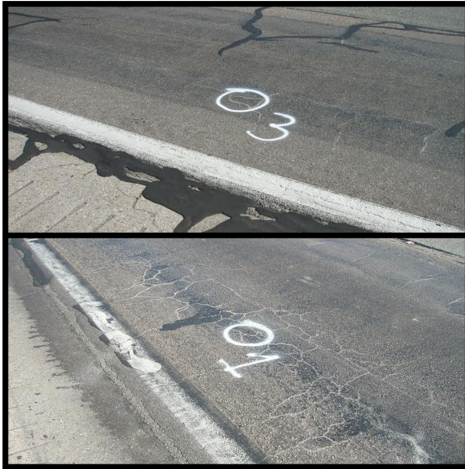
Figure 3.4: Low (Top) & High (Bottom) Severity Alligator Crack
