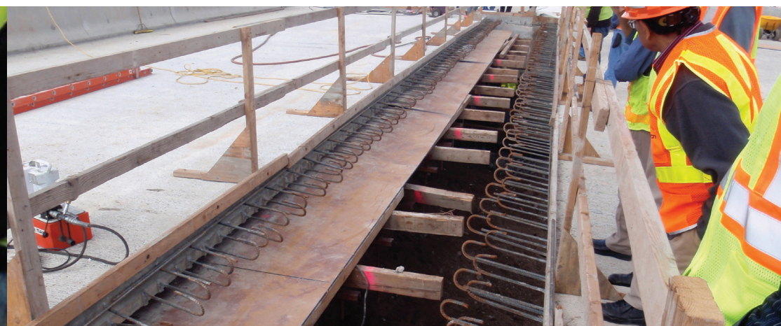
Hydraulic pumps help slide the new and improved Gila River Bridge (Str. 145) in place significantly reducing the long detour caused by the bridge closure for the Gila River Indian Community in Sacaton, Arizona. Photo courtesy Nenad Gucunski
