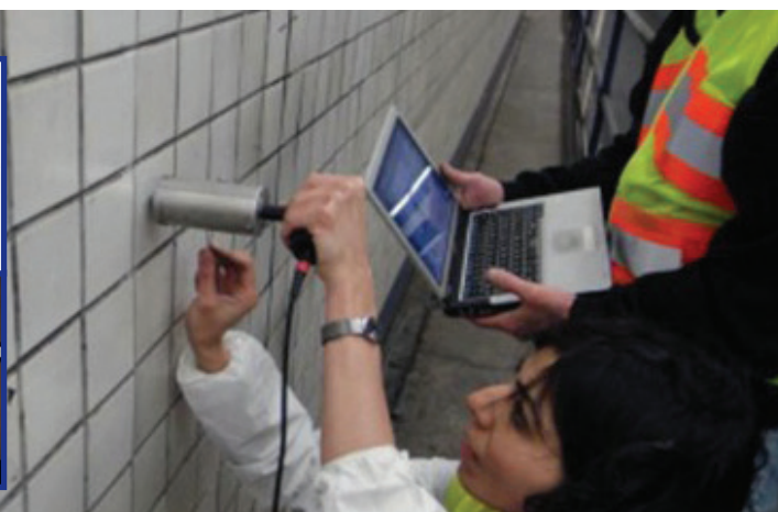
State participants gather to observe hand held (or various types of) NDT equipment testing on tunnel infrastructure. Photos courtesy Texas A&M University
