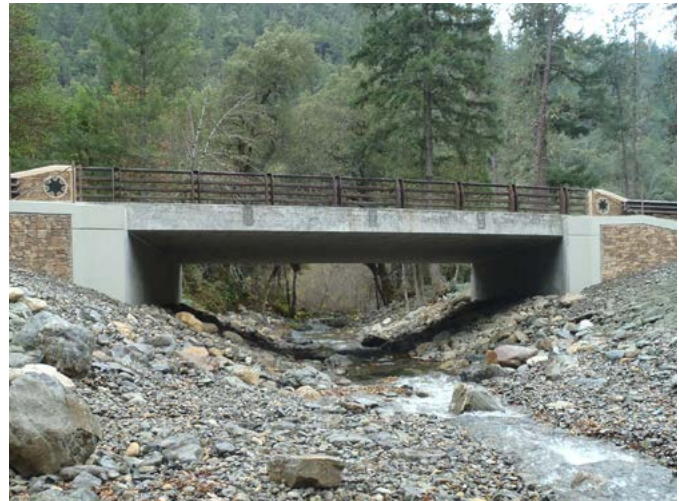
Caltrans used Innovative Bridge Designs for Rapid Renewal (R04) in the renewal of the Fort Goff Creek Bridge.
