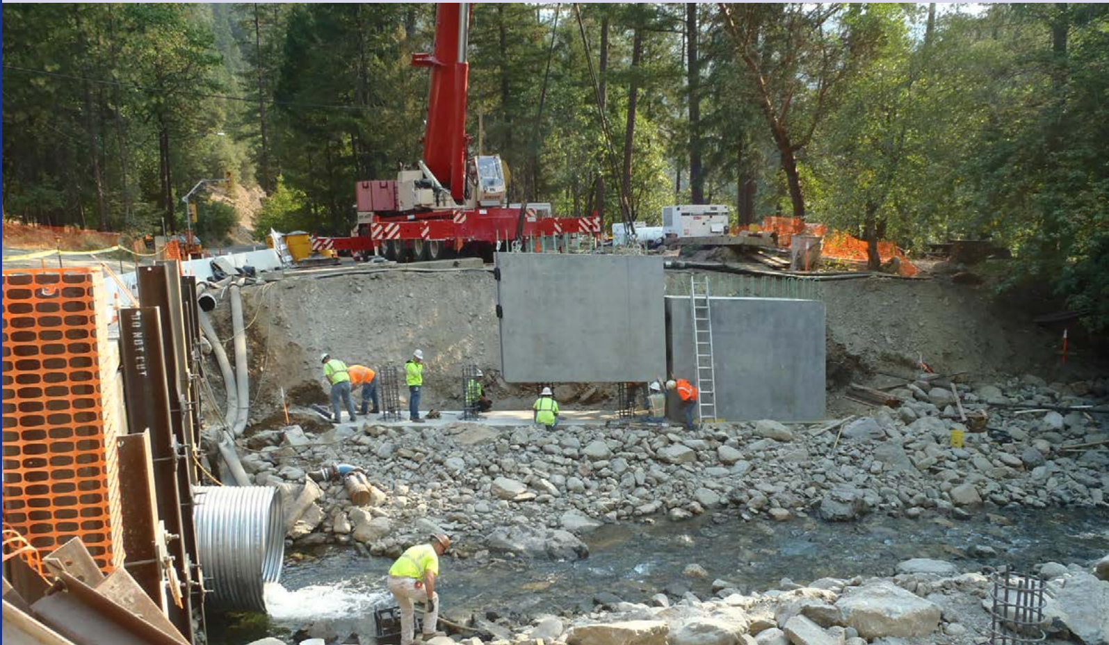
Fort Goff Creek Bridge – placement of 85-kip abutment segments Source: Accelerated Bridge Construction Center at Florida International University
