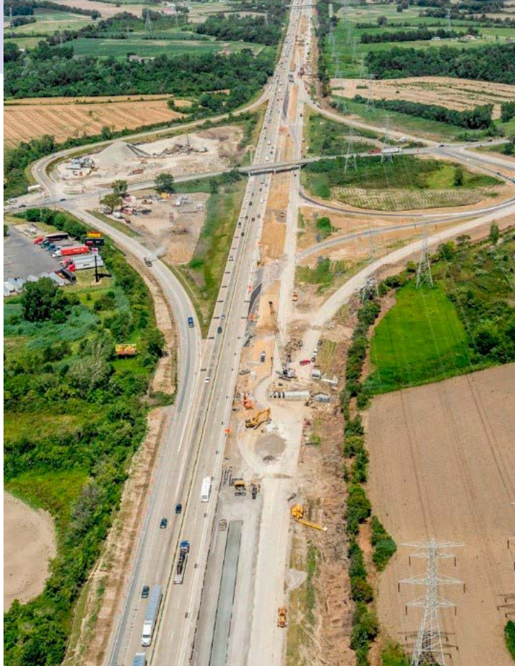
I-75 in southeast Michigan near Lake Erie. Source: Michigan Department of Transportation
