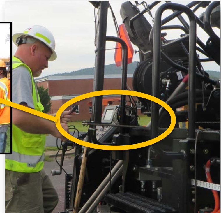
Mounted to a Steel Plate Attached to Work Platform
