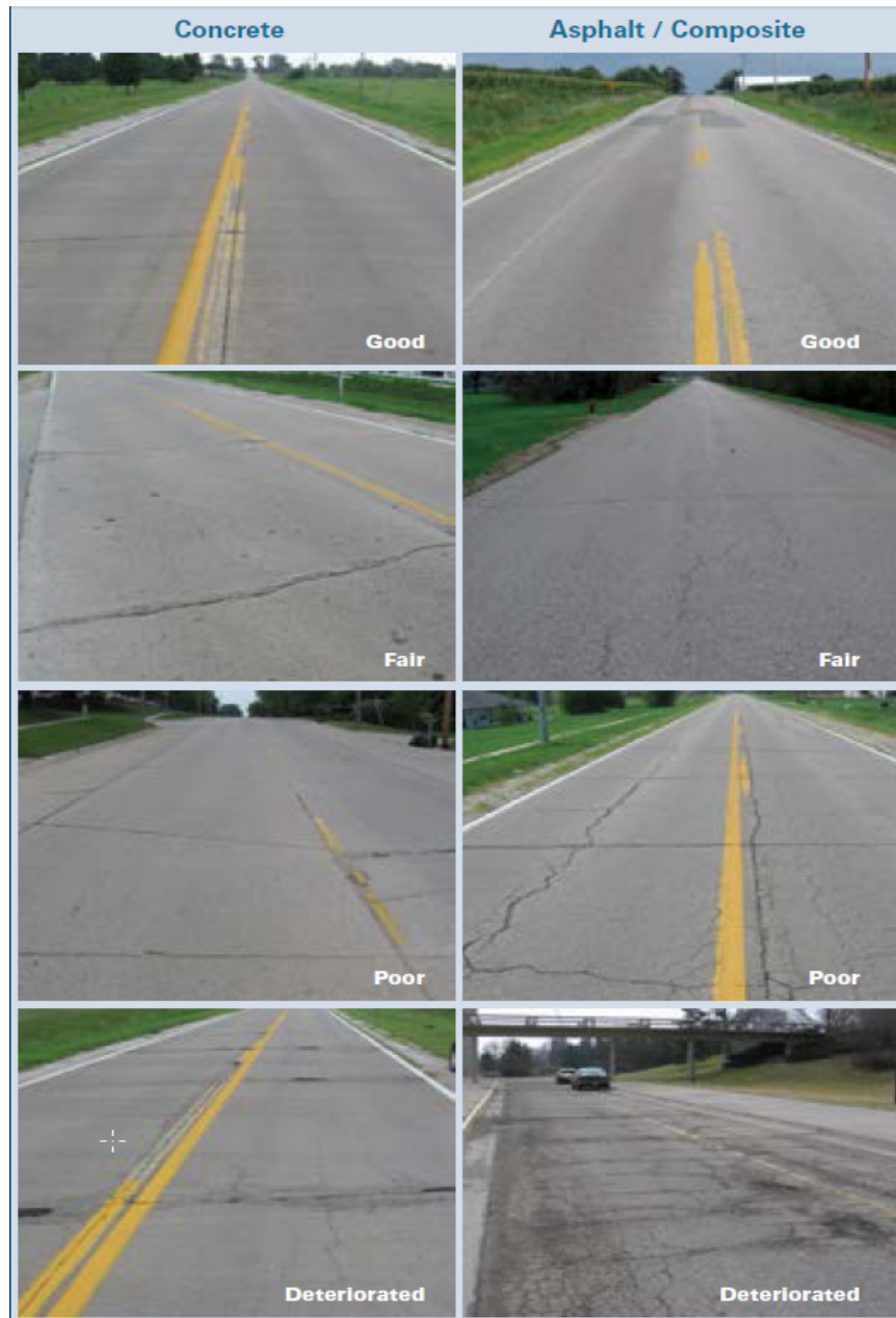
Figure C-1. Example Illustrations of Overall Pavement Condition (Harrington and Fick 2014).
