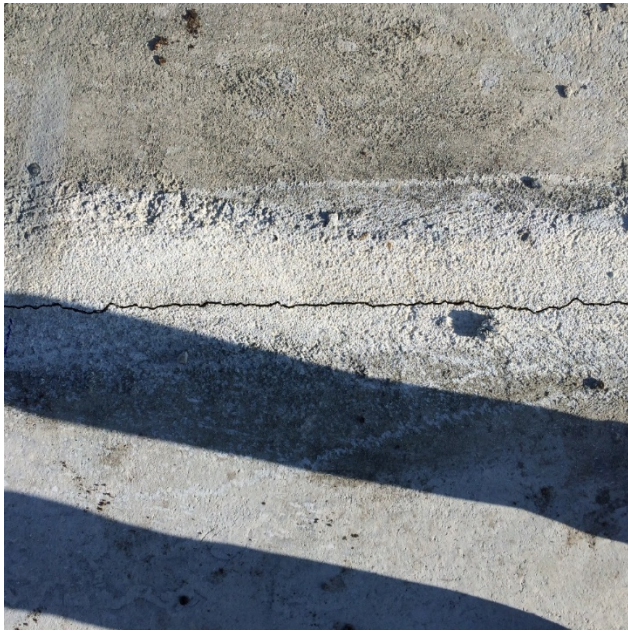
Before Post-tensioning Crack width = 0.086 in.
