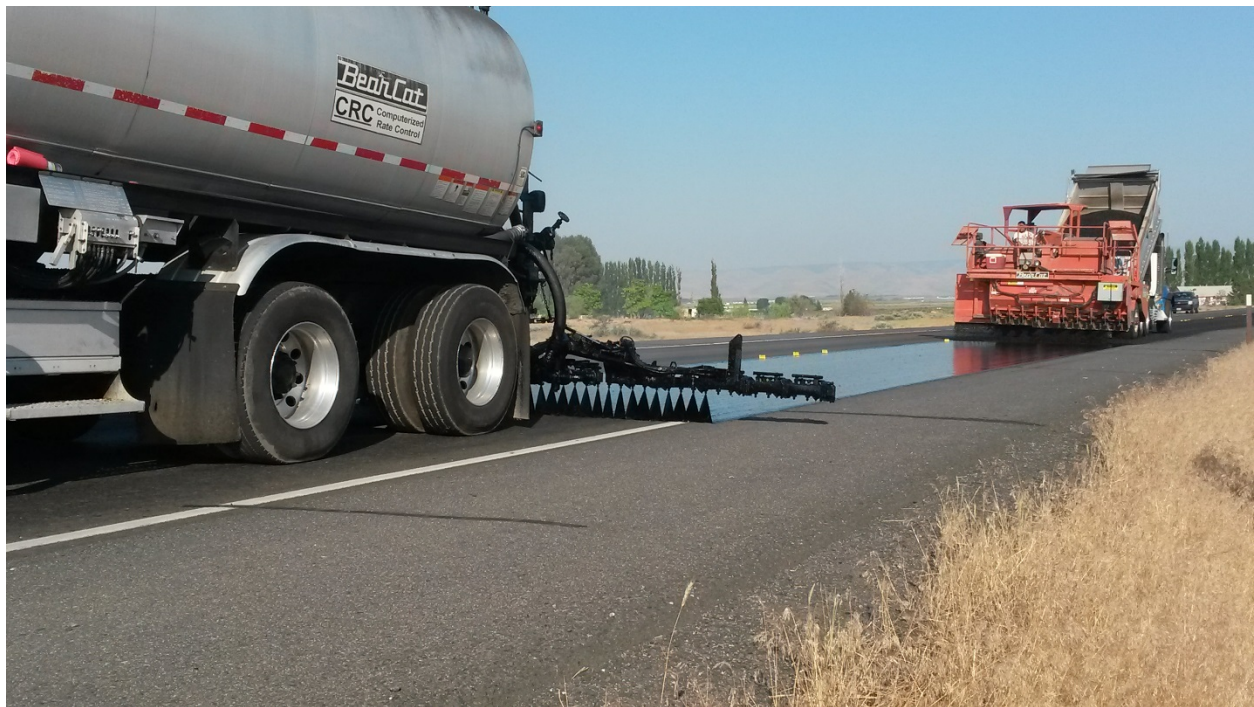
Figure 1. Hot-applied asphalt cement provides the adhesion for chips to the pavement surface.
